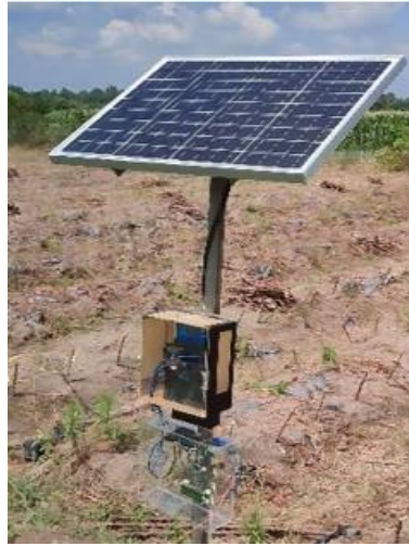
Figure 2. overall solar PV
