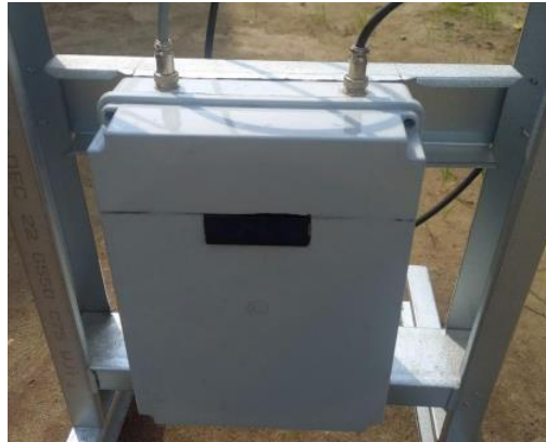
Figure 3. Solar Tracker Box Panel
